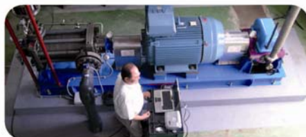
Cangrejo T.M desalination plant, Valverde - El Hierro- Canary Islands.
