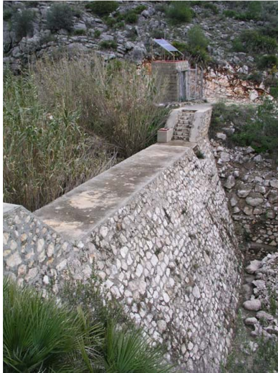
Figure 8. Most of the MAR volume stored in Spain (estimated about 380 hm 3 per year) is “accidental” by means of dikes and little dams upstream basin areas.
