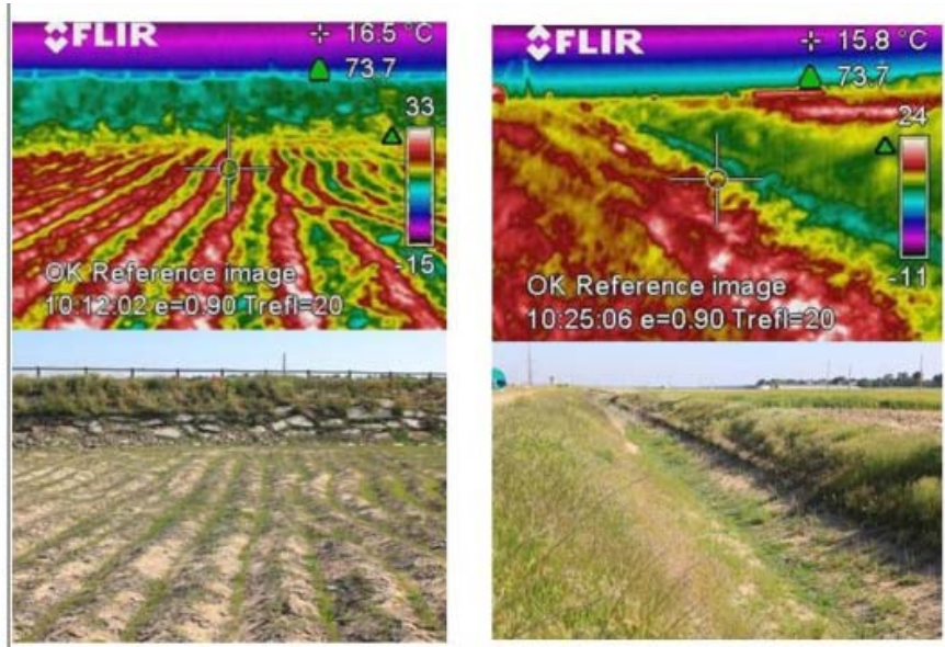
Figures 12. Comparison between normal and thermographic aspects, in order to allocate clogging processes.
