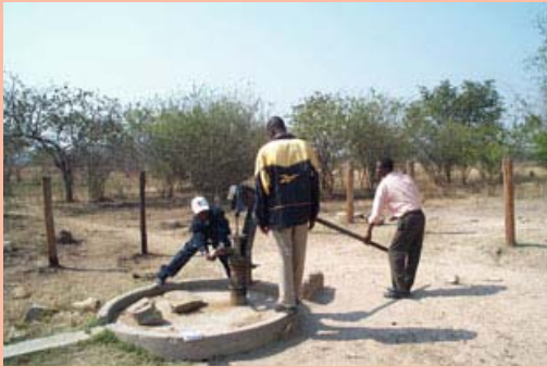
Box Fig. 3.3a.1 Testing a faulty borehole during Zimbabwe's dry season in 2000. Boreholes are the main supplier of water in the rural areas (Photo credit: William Derman)
