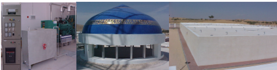
Photos of Phase 1: Jaalan Bani bu Hasan and Jaalan Bani bu Ali Scheme
