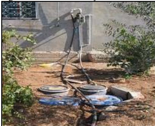
Figure 1. Four-Barrel Greywater Treatment Unit
