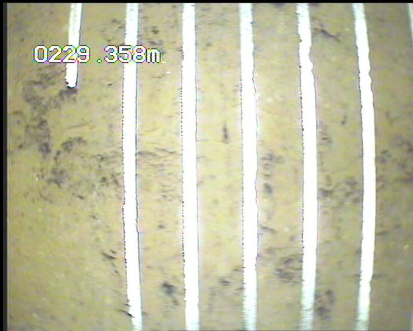
Poor mud control and development resulting in clogging of screen
