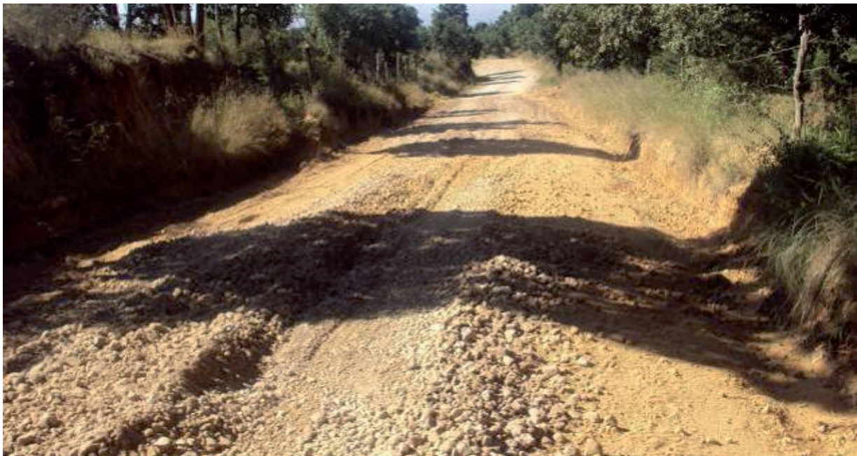
Figura 4. Mantenimiento del camino principal de acceso al bosque. Figure 4. Maintenance of the main access road to the forest.
